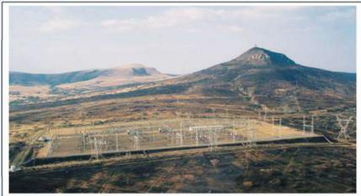
Figure 16: Overview of the substation.
