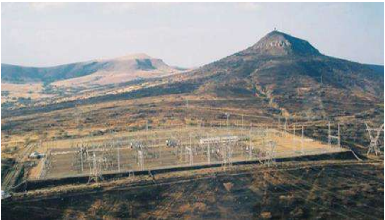
Plate 1: showing Umfolozi Substation where the proposed powerline will connect(Photograph by Menno Klapwijk)
