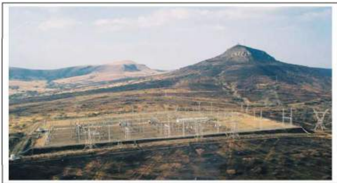
Figure 7: Overview of the substation
