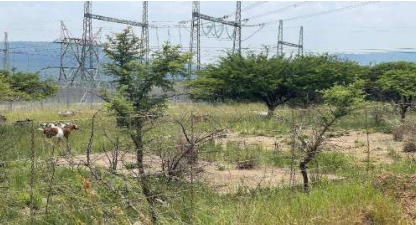
Plate 2: showing the Umfolozi Substation
