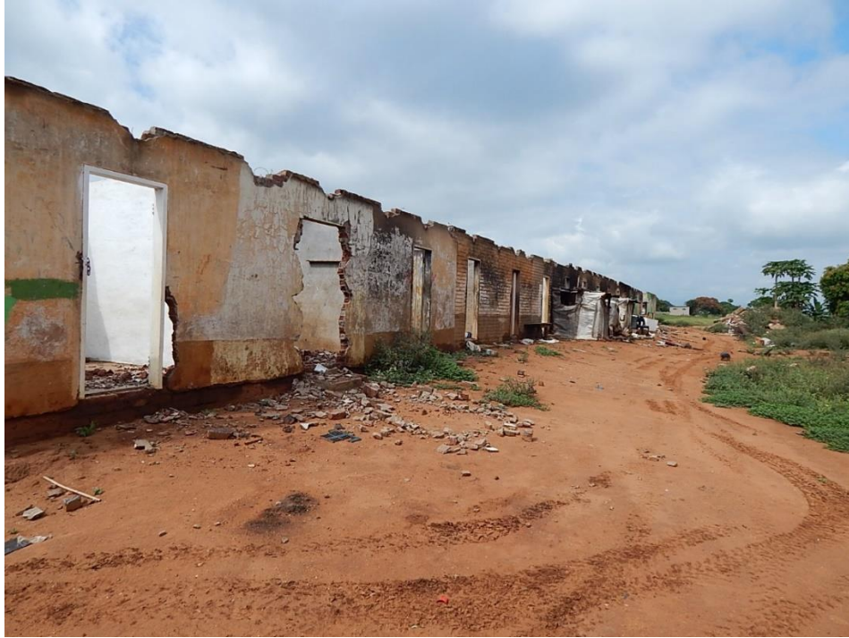
Fig. 27: Previous farm workers accommodation (compound) in the northern section, which is now derelict.
