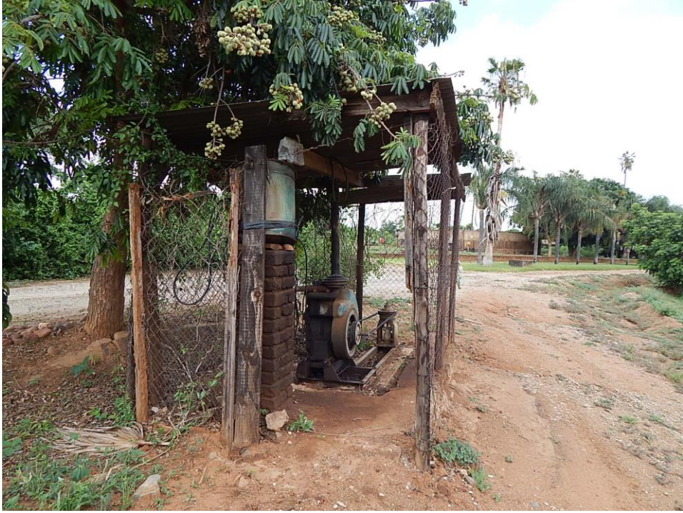
Fig. 21: Another pump for use on the farm.
