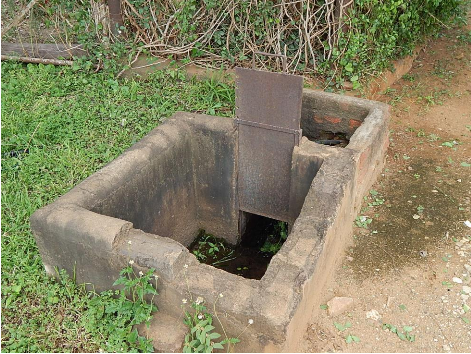
Fig. 23: A few small weirs are visible near the farm residence, to regulate water into the canals.
