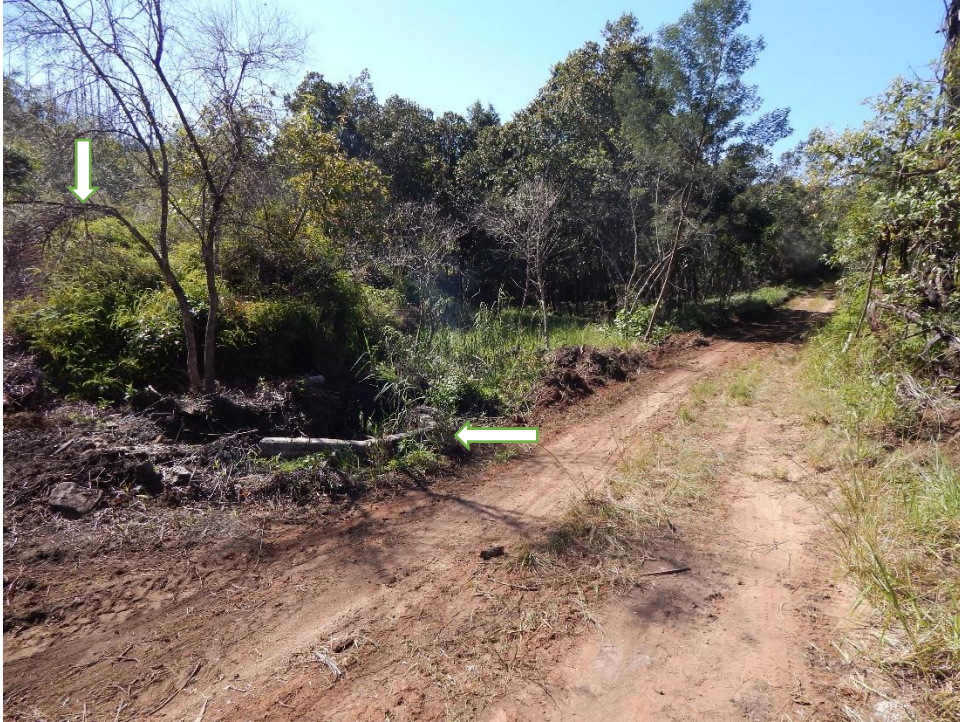
Fig. 10: Weir 2 will be constructed from the low outcrop to the left (see arrow), to incorporate the stream which flows under the gravel road (see arrow).
