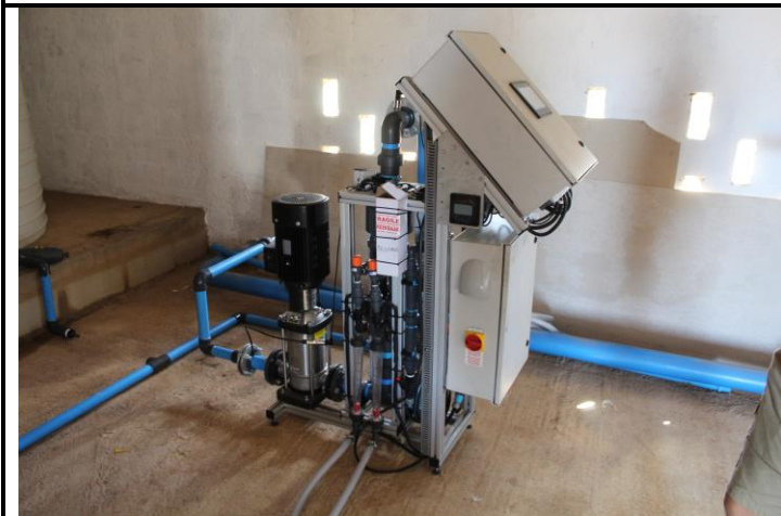
Figure 11: Pump houses and irrigation systems are in place and functional.
