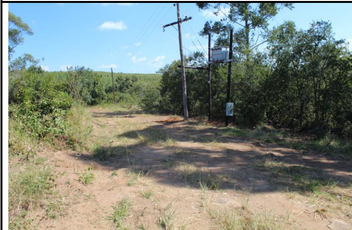
Figure 17: Eskom Facility: Functional and upgraded with adequate capacity.
