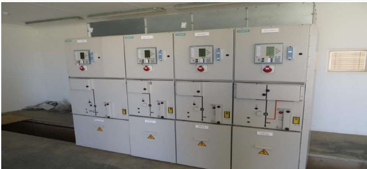
Figure A13: MV substation (inside)
