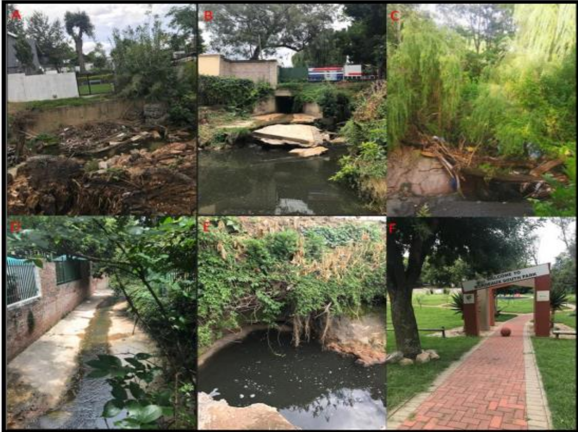
Fig: Indicating some of the impacts identified during the site assessment: Frame A: bank stabilization; Frame B: Calvert under Main Road; Frame C: Woody vegetation, debris and litter; Frame D: Canalization of sections of the channel; Frame E: Active erosion within the channel; Frame F: Bordeaux South Park in a historical valley bottom wetland system (Rose Garden Park and the Denise Park are located up gradient of the study site within the same wetland system).
