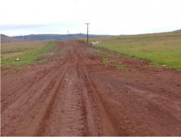
Photo 11: Road is traversing the seep wetland
