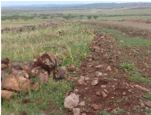
Photo 5: Old House foundations damaged
