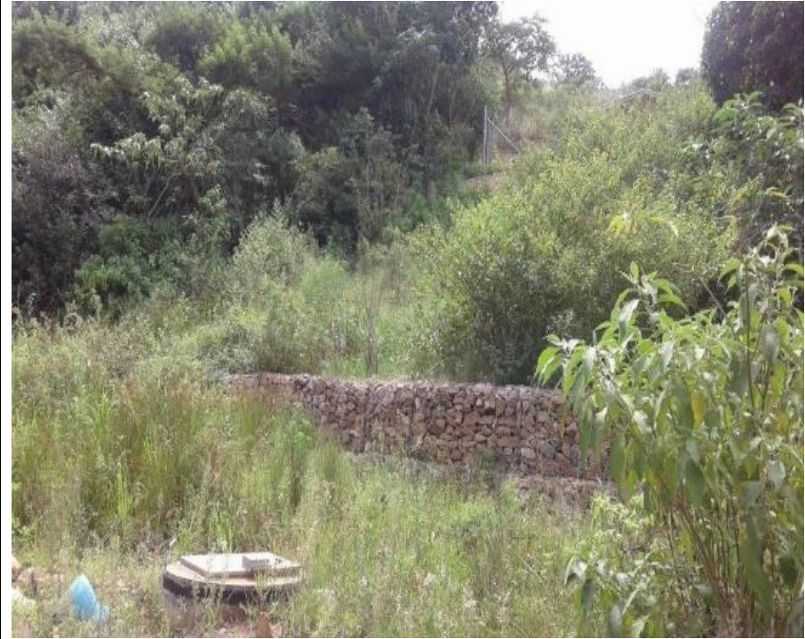
Photo 2: View of the gabion retaining wall below the outlet pipe which are acting as a control to minimise erosion caused by the discharge of water from the raw water pumphouse.
