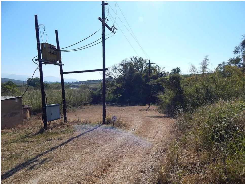
Fig. 20: The north-western corner where the dam wall will be situated. Please note the large powerlines and pump station (farm ESPERADO ANNEX).
