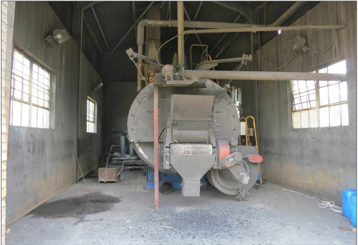
Figure 7: One of two coal fired boilers used to generate steam on site
