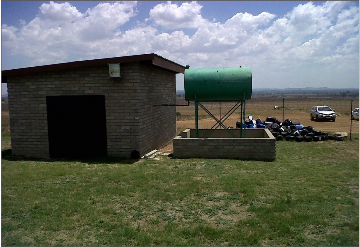
Figure 5: Backup generator and bundled diesel storage tank
