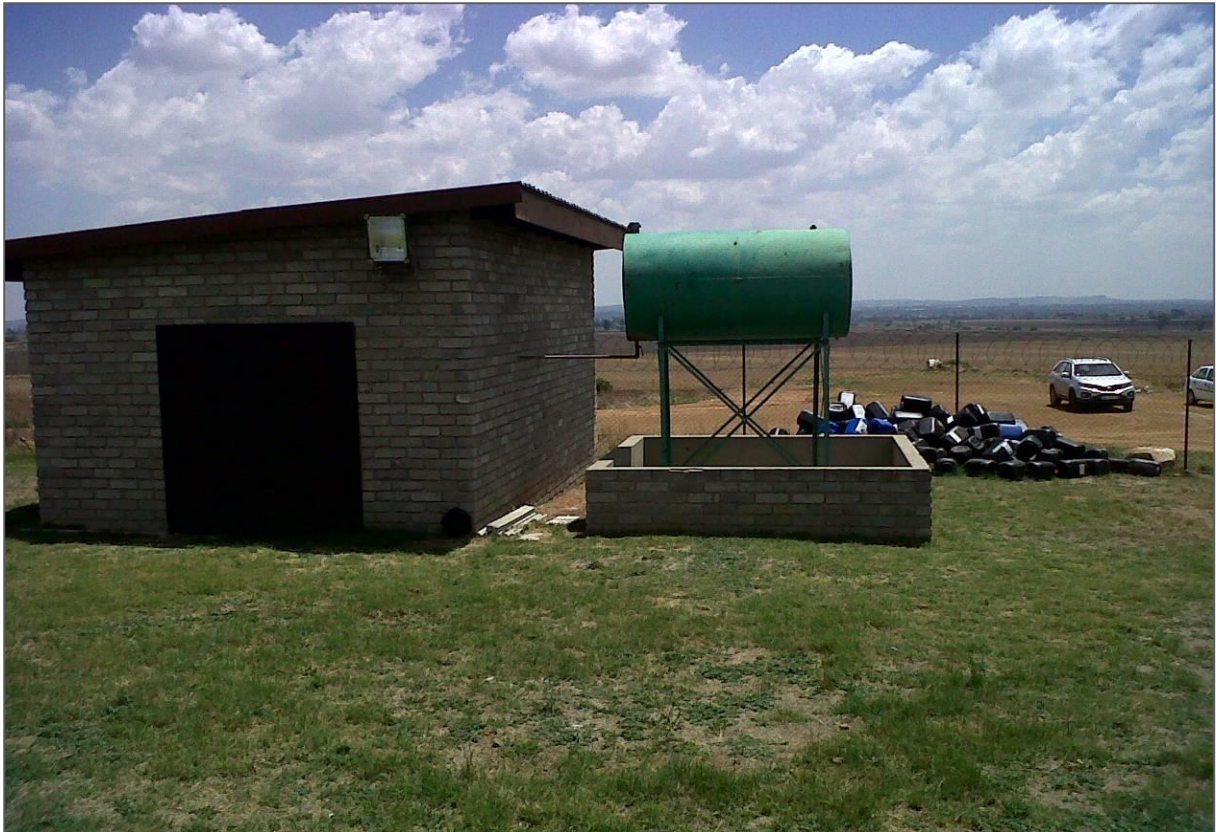
Figure 5: Backup generator and bunded diesel storage tank
