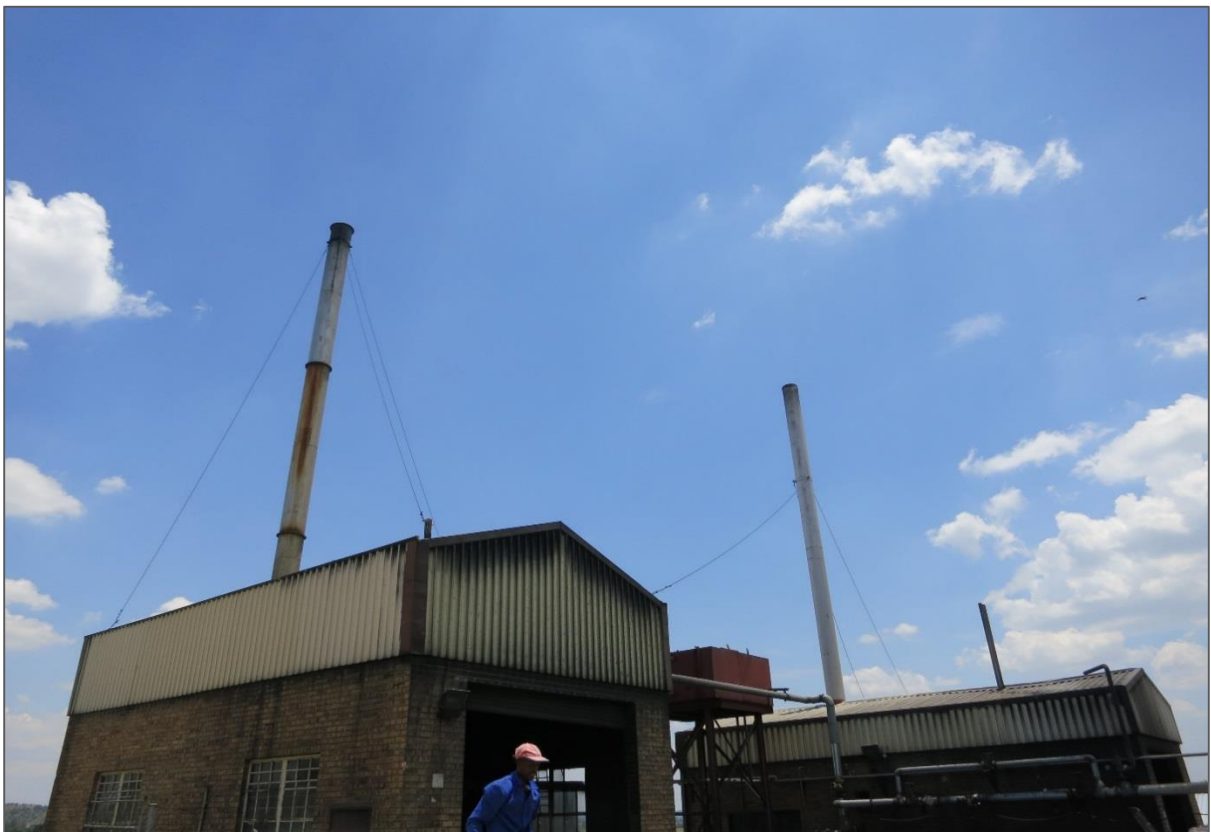
Figure 8: The two boiler stacks
