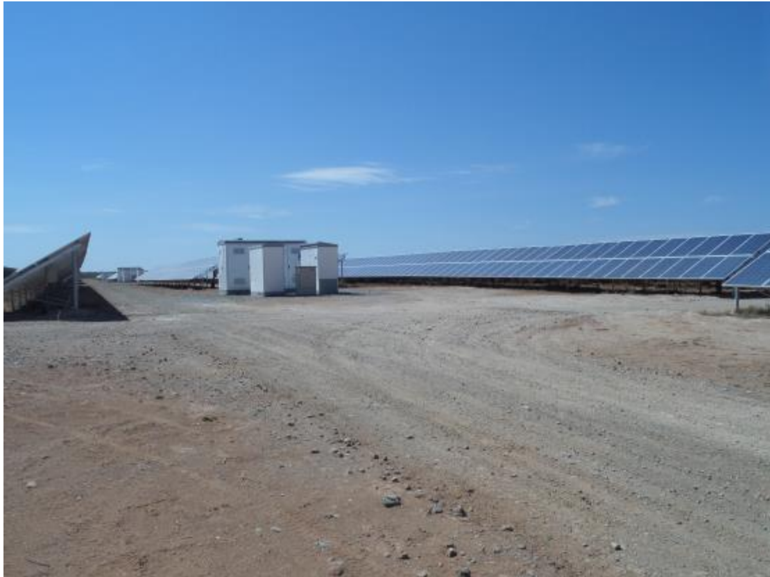
Fig 8 Image depicting fixed PV modules with inverter (source SDP)
