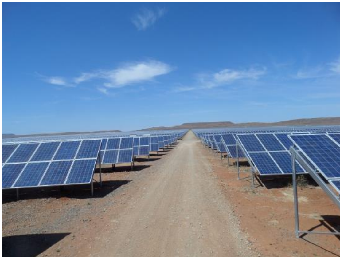
Fig. 4 Image indicating the nature of a fixed PV park and module arrangement
