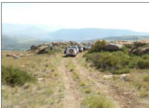
Figure 10-16: Resistant caprock in roadbed.
