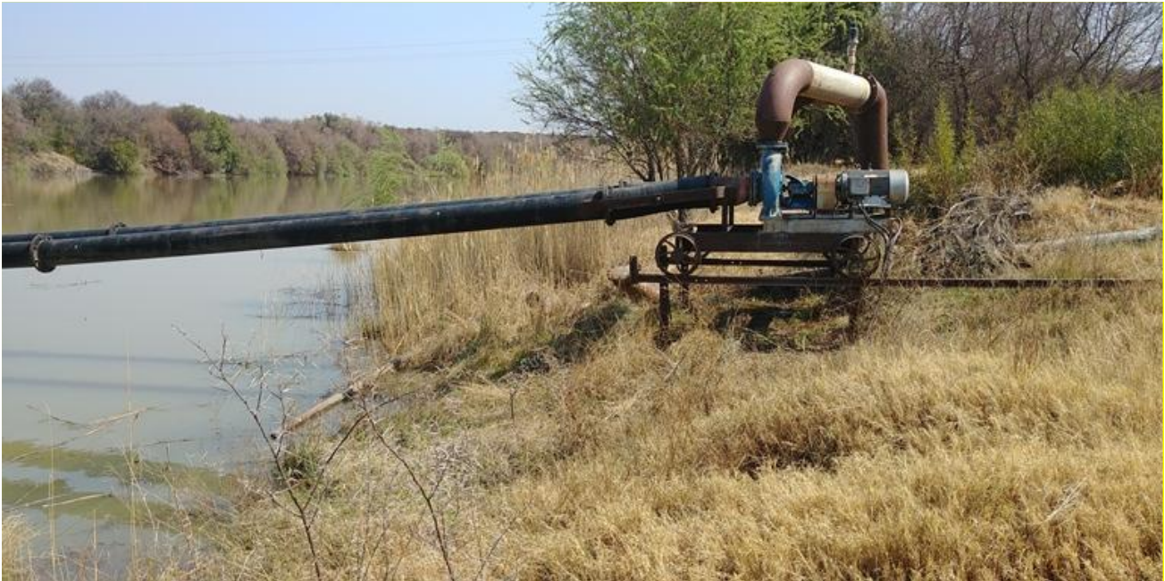
Figure 12: Image illustrating the presence and narrow, confined impact of the pumping infrastructure
