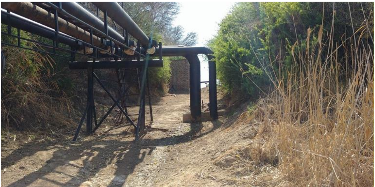
Figure 14 a & b: Two images illustrating the presence and narrow, confined impact of the pumping and associated piping infrastructure
