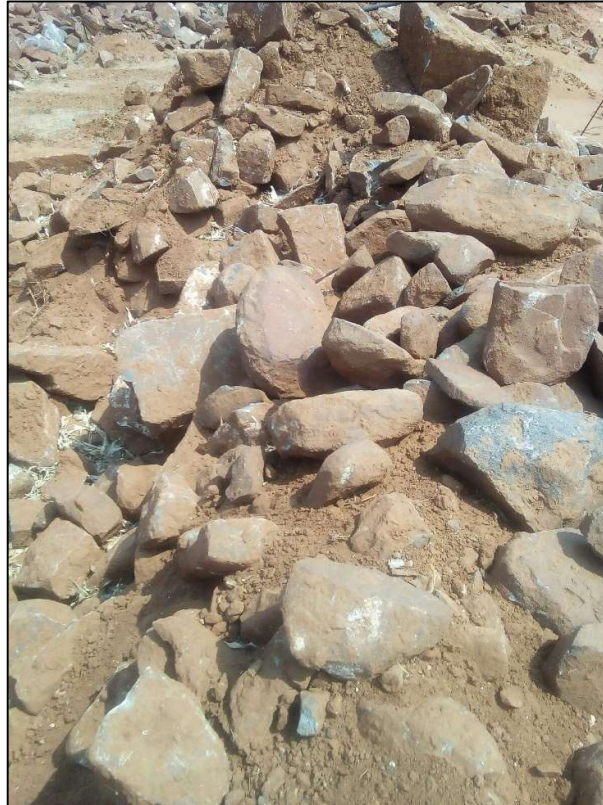
Figure 10: Loose boulders which is the limiting layer in the shallow southern area.
