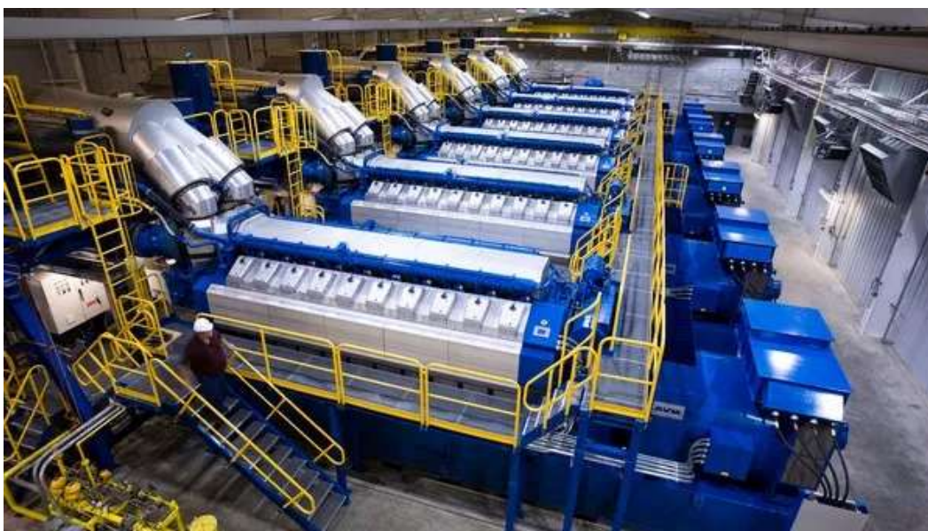
Figure 3.4: Engine Hall of typical Gas Engine power plant
