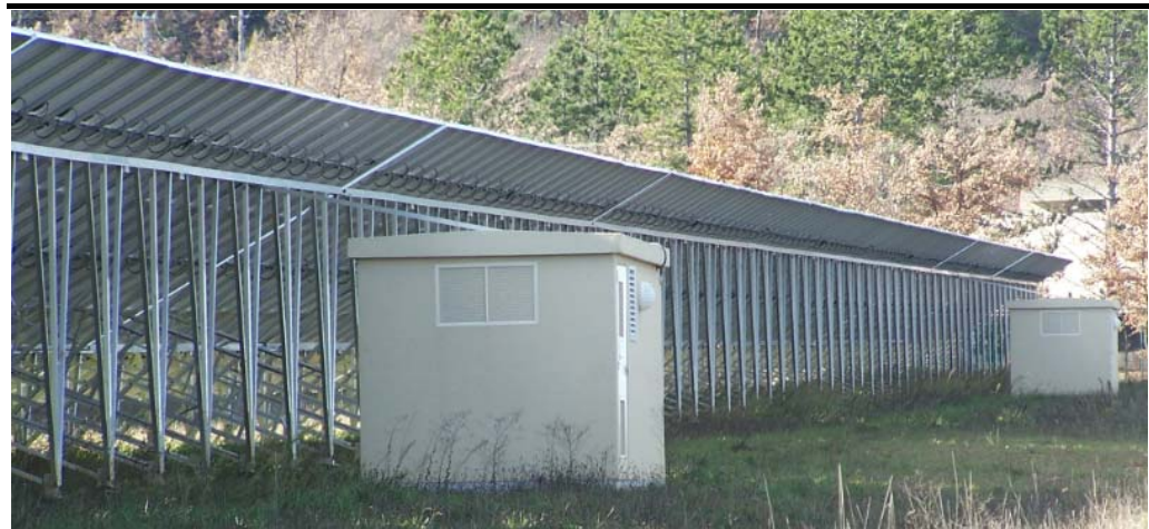
Figure 4.7 Typical Inverter/Transformer Enclosures
