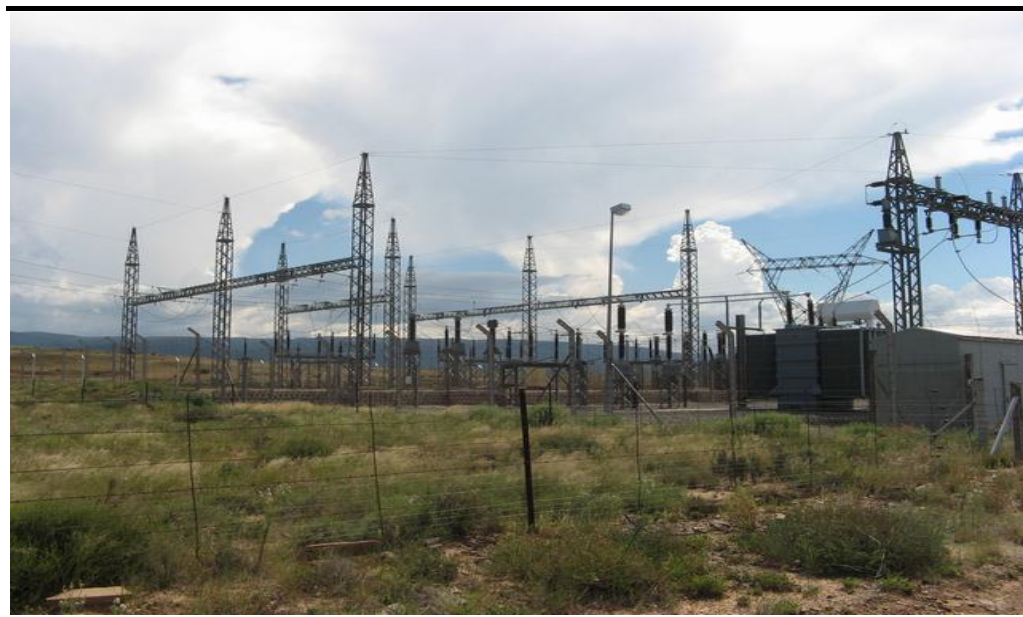
Figure 4.10 Existing Drenman Traction Substation
