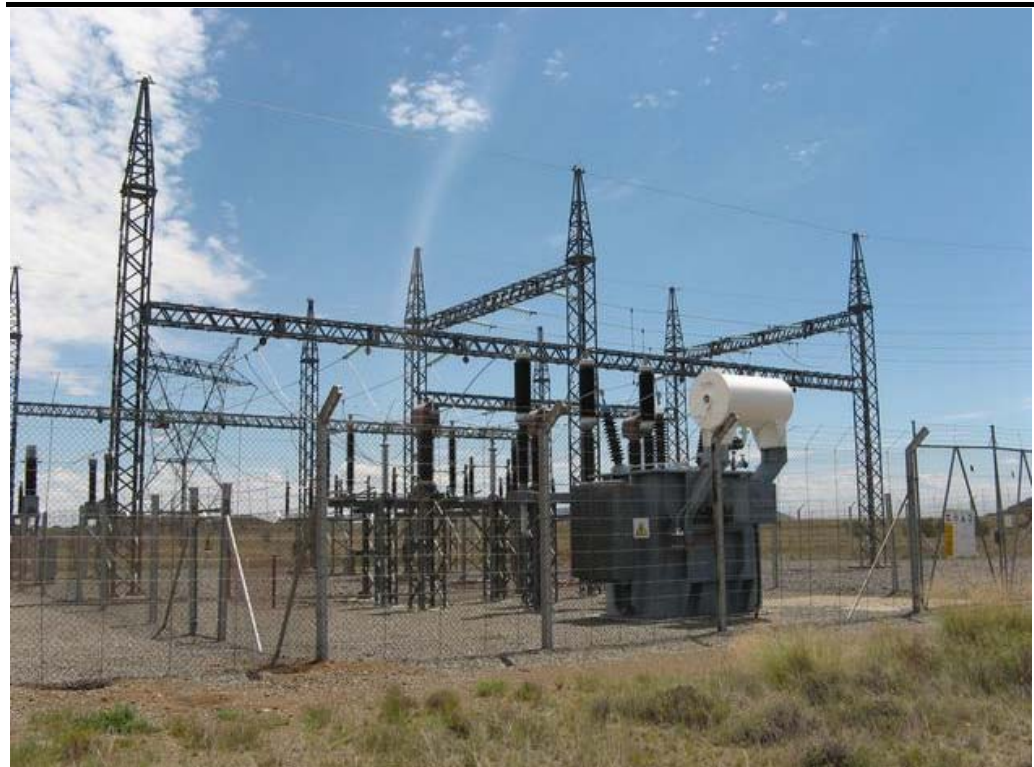
Figure 4.9 Transformer in Grid Connection Substation Yard
