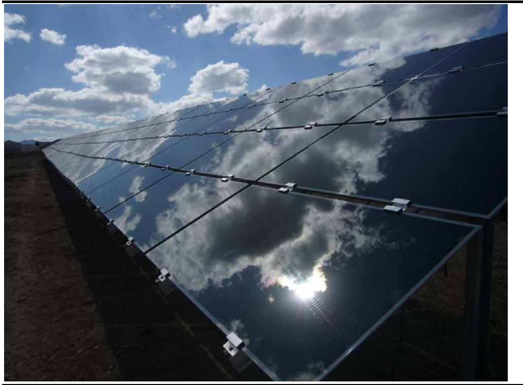
Figure 4.4 Typical PV Array
