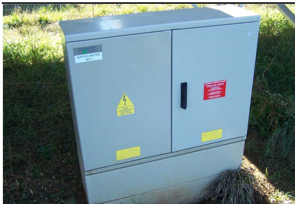
Figure 4.5 Typical Array Enclosure
