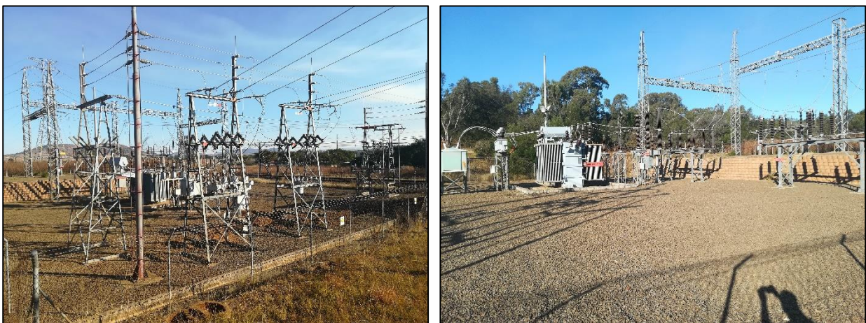
Images 3: Dannhauser 88/11kV, 10MVA Substation
