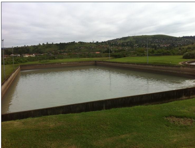
Photo 3: The existing balancing tank
