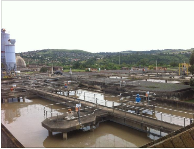
Photo 1: The existing anaerobic reactor to be converted to a RAS conditioner
