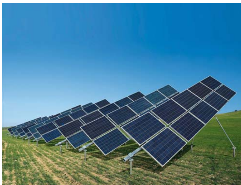
Figure 3.11: A Polar Tracker mounted system (from RV & Associates).
