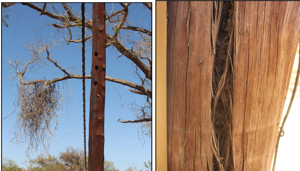
Figure 2: shows the problems associated with the existing poles which have introduced challenges associated with load strain from the powerline. This poses a strong risk to human and animal life and must be urgently addressed.
