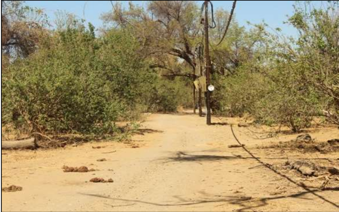
Figure 10: Electrical route alongside the gravel road
