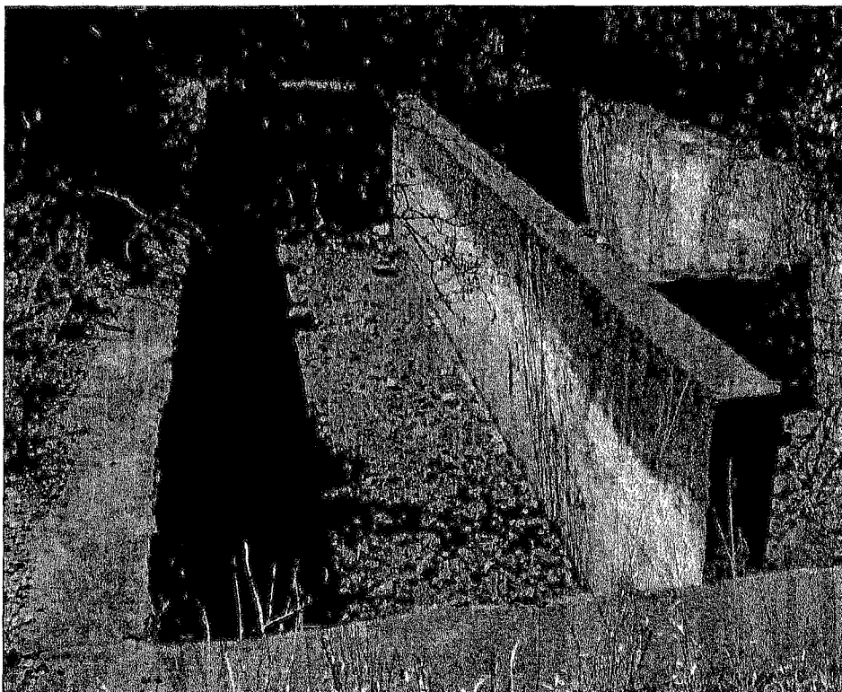
Fig.12 Concrete lined pit with dividing wall down the centre. Note water line on the wall.
