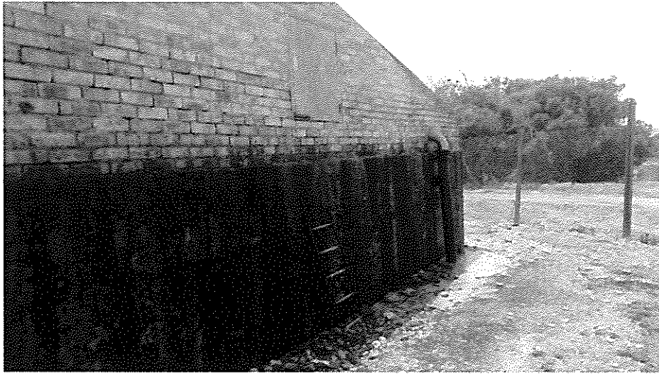
Figure 5-5 Seawater reservoir overflowing
