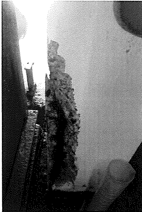
Figure 5-9 Exposed reinforcement on columns
