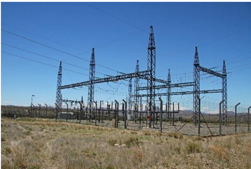
Figure 9: The proposed development site already houses the Eskom Dobbin sub-station next to the railway line.
