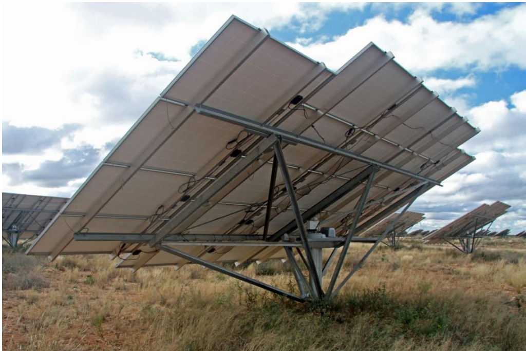
Figure 15: A dual axis tracker PV solar mounting
