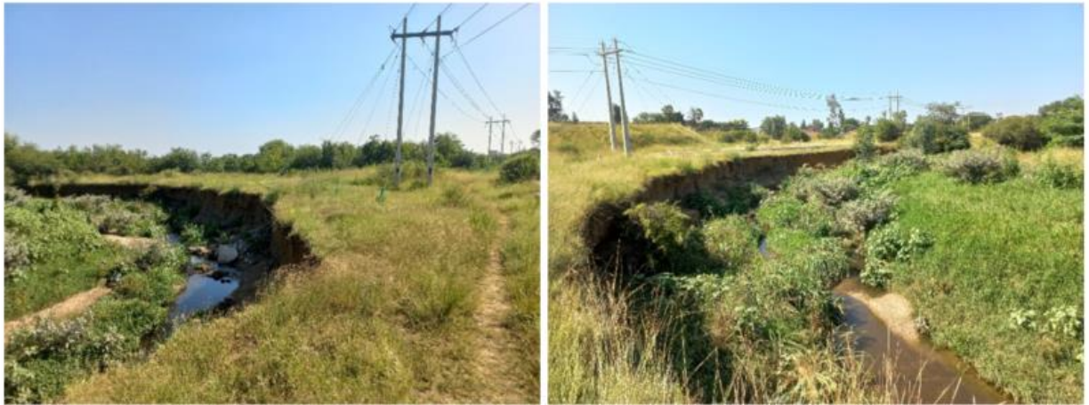
Figure 5-10 Photos showing the eroded riverbank and the proximity of the adjacent powerline poles and stays (WCS Scientific, 2022)
