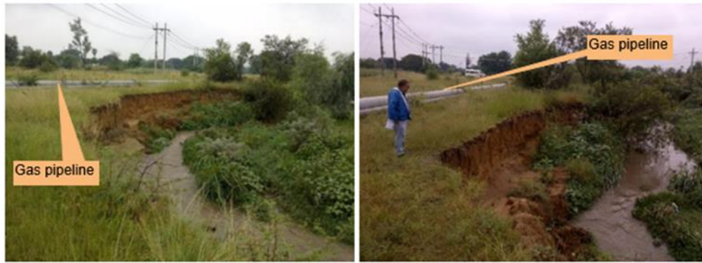
Figure 2-2 Gas pipeline ≈5m from the riverbank (HEES, 2022)
