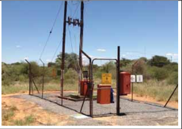
S1 – Transformer Yard
