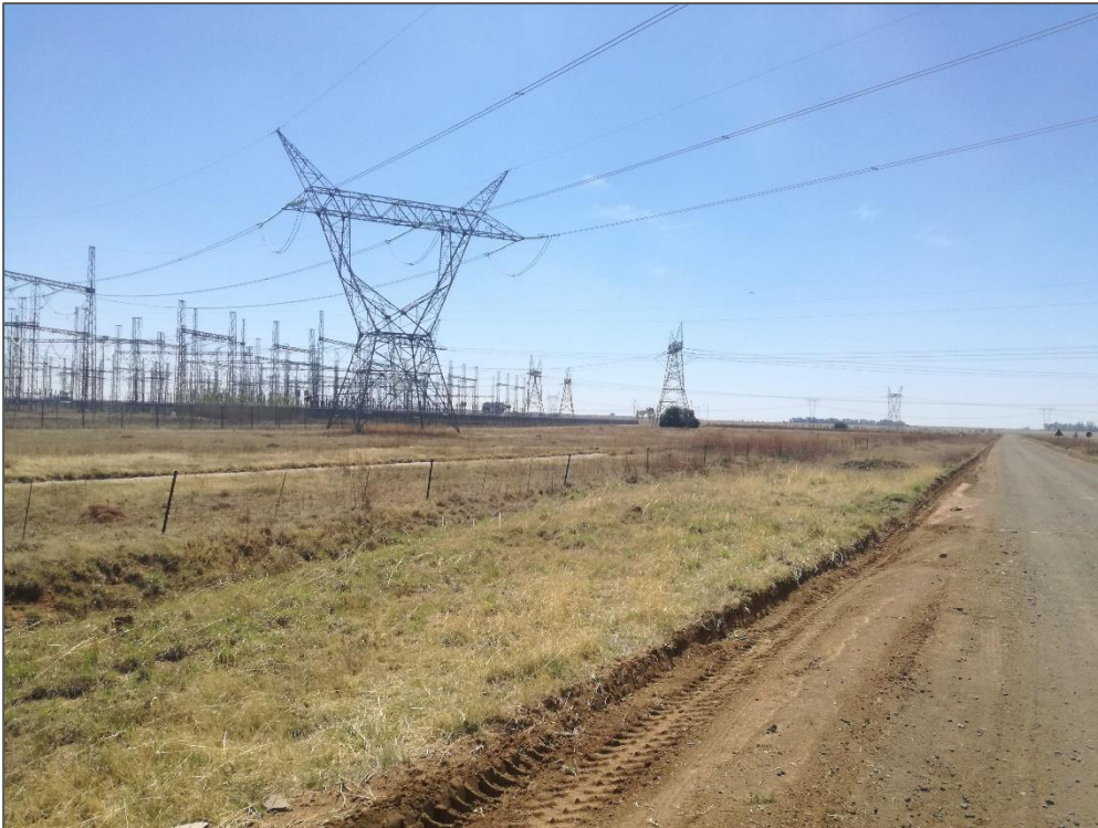
Figure 7-39: High voltage power lines feeding into Perseus Substation.
