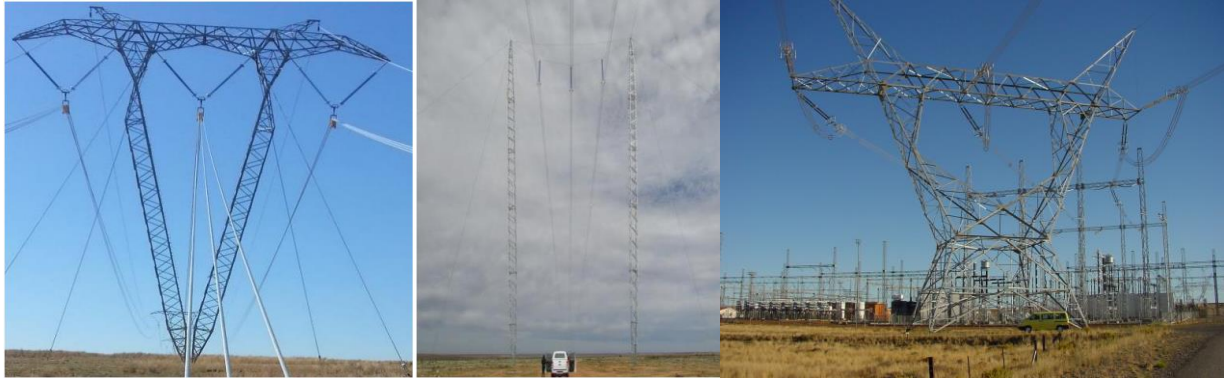
Figure 4-3: Typical 400kV Gayed V type (left) and Cross-Rope suspension (middle) and self-supporting (right) design
