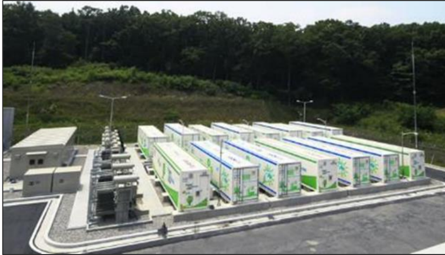
Figure 4-4: Example of a Lithium-Ion BESS installation
