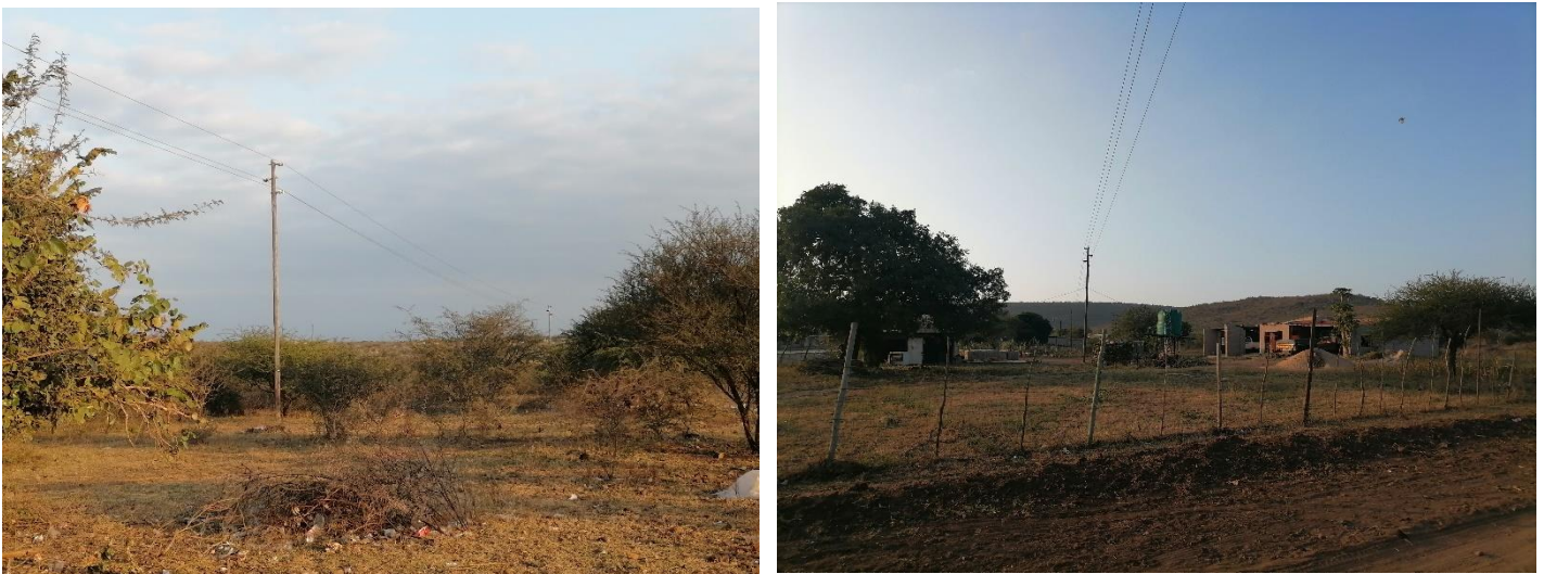
Figure 34: Eskom Power Lines (Site Visit, 2023)
