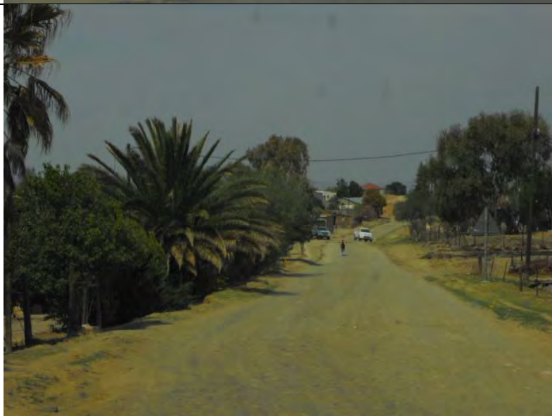
Figure 9: View of the Phase 1 pipeline along the western split. The pipeline will be installed adjacent to the road.
