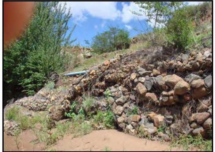
Figure 15: Gabions collapsed at river bank
