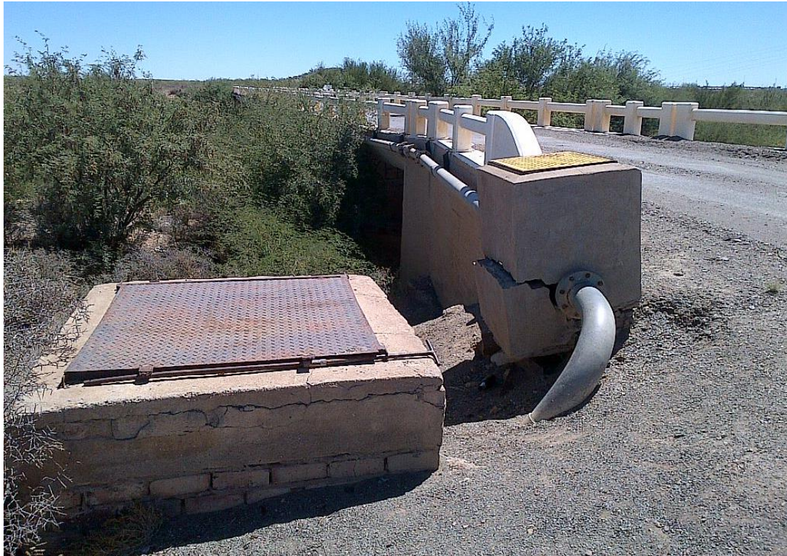
Figure 6: Bridge crossing over Sak River. As in the photograph above, the proposed pipeline will be attached to the bridge
