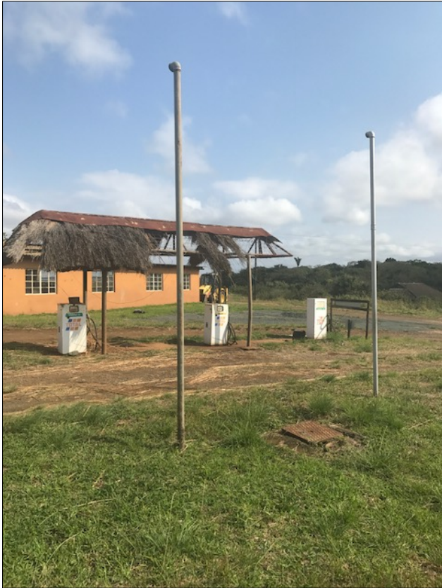
Photo 2: Pump islands with vents for tanks 1 and 2 in the foreground
