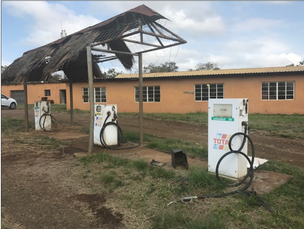
Photo 3: Image showing the current condition of the pump islands and canopy with workshops in the background
