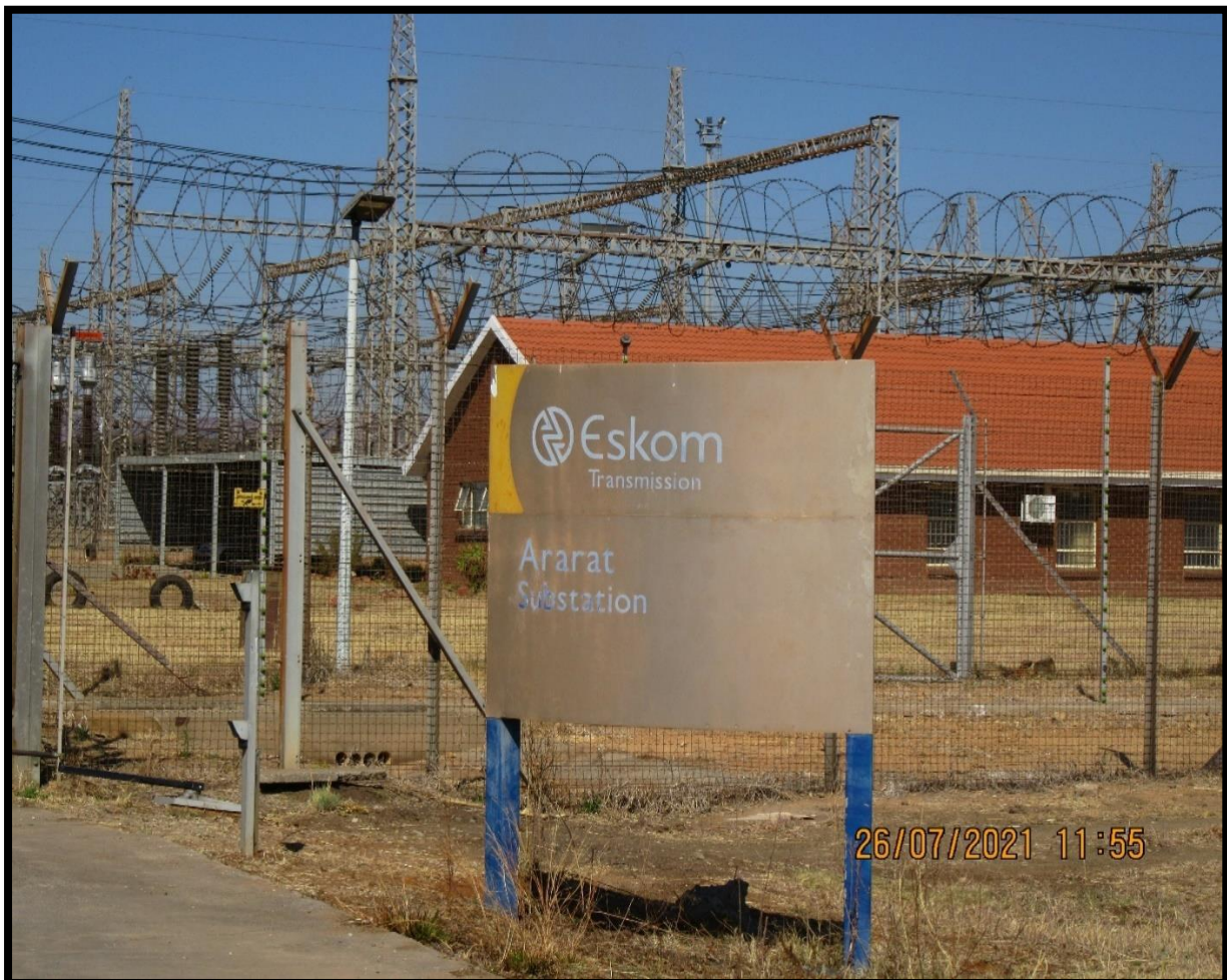
Figure 7: Entrance to Ararat Main Transmission Substation
