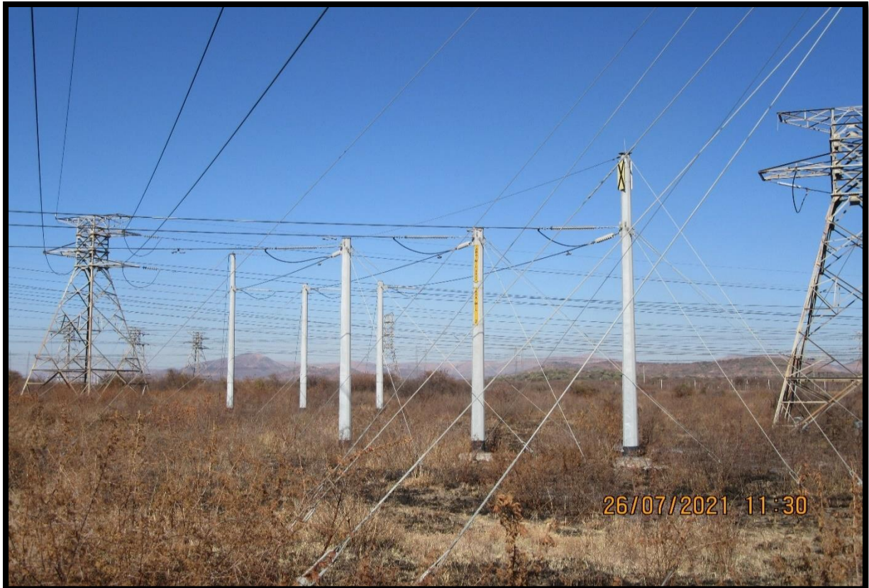
Figure 9: Existing low-lying D-DT 7618 tower structures taking power from Ararat MTS which are proposed for Ararat Alternative Route A
