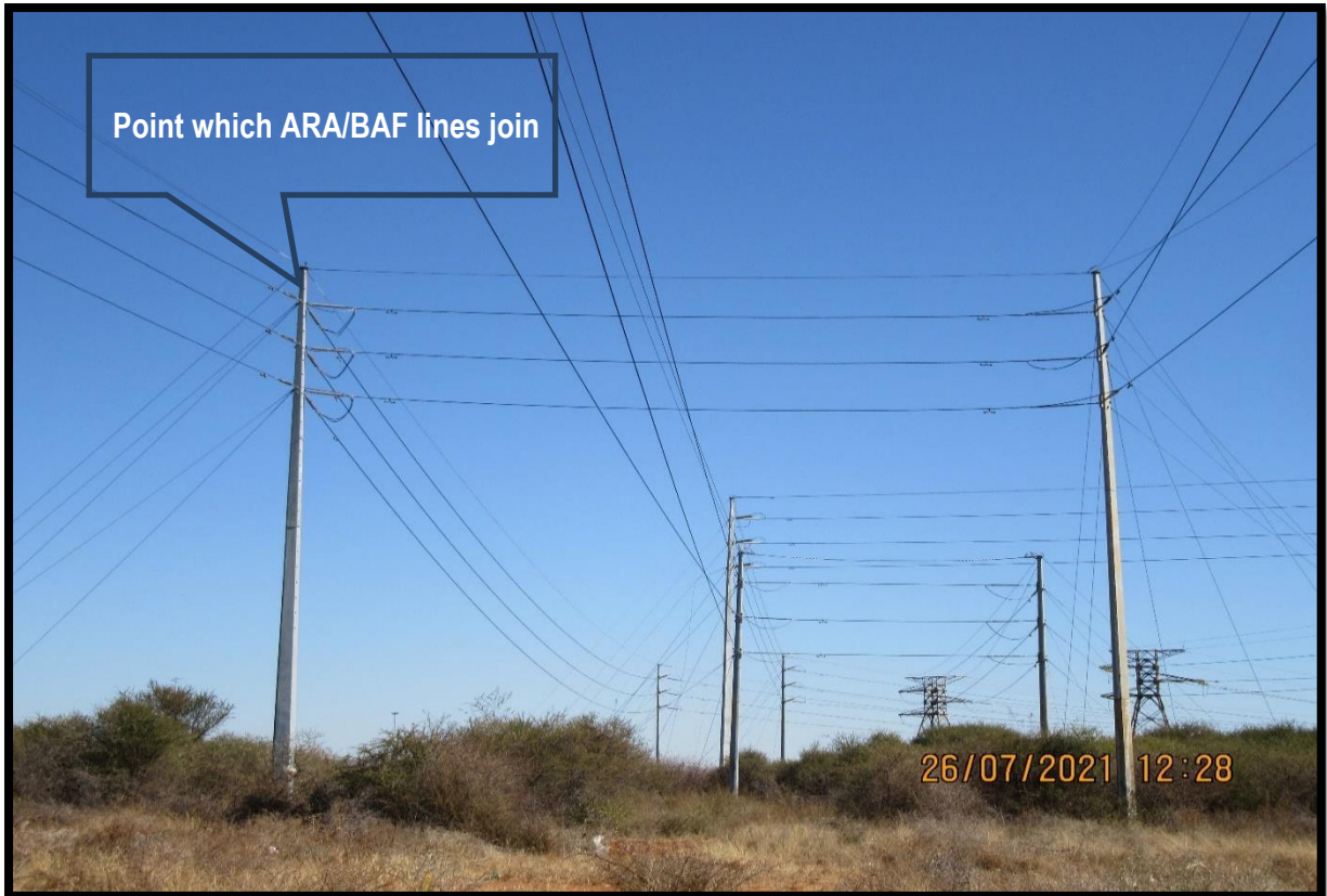
Figure 12: Image showing point at which the ARA/BAF lines from Ararat MTS join into one single line into Bafokeng 7 substation
