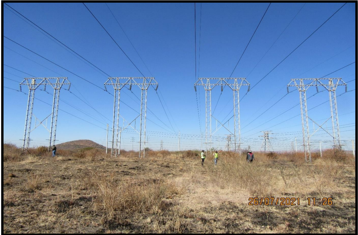
Figure 8: Separate Ararat-Bafokeng (ARA/BAF) lines (middle two) after conjoint out of Ararat MTS
