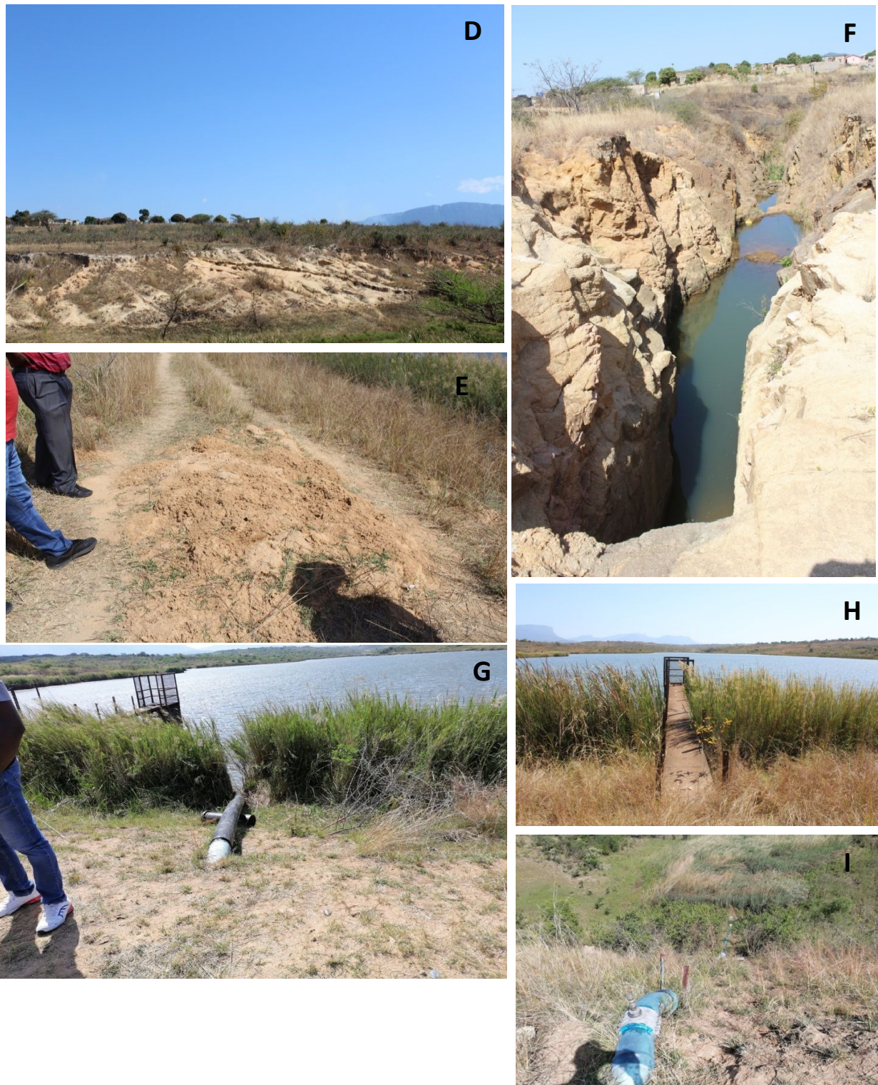
Plate 3: (D) Erosion along the right flank of Casteel Dam; (E) Termites colonising the dam wall/crest, (F) Large donga in the spillway channel; (G) Intake tower (metal/iron parts removed overtime making it unsafe (H) & (I) Temporary pipeline over the dam embankment releasing water to downstream water users.
