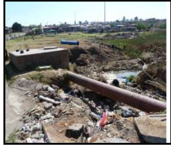
Figure 2: Excessive illegal dumping at Kalkspruit Bridge
