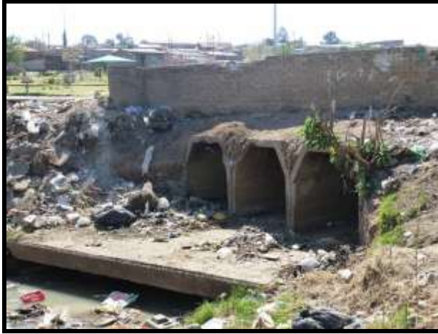
Figure 1: Existing undermined bridge structure
