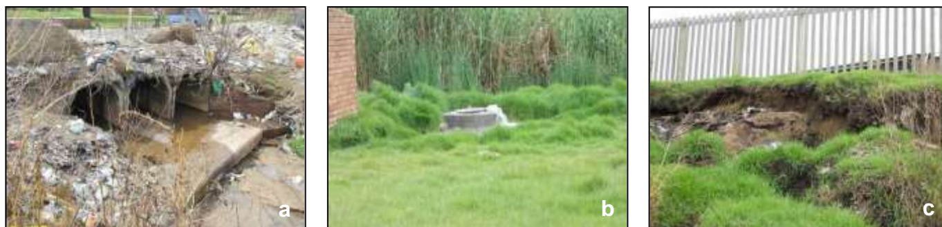
Figure 8: (a) litter and illegal dumping in the stream, (b) blocked sewerage drain overflowing into wetland and (c) erosion of stream banks
