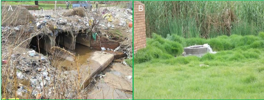
Figure 11: A) Illegal dumping of waste material by the local community and B) the blocked sewerage drain overflowing into the wetland system.
