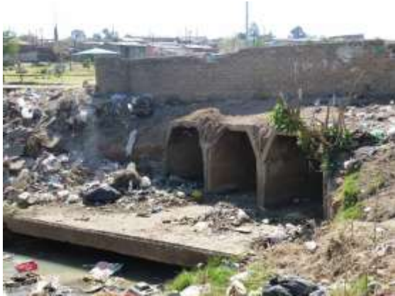
Figure 2: Existing undermined bridge structure
