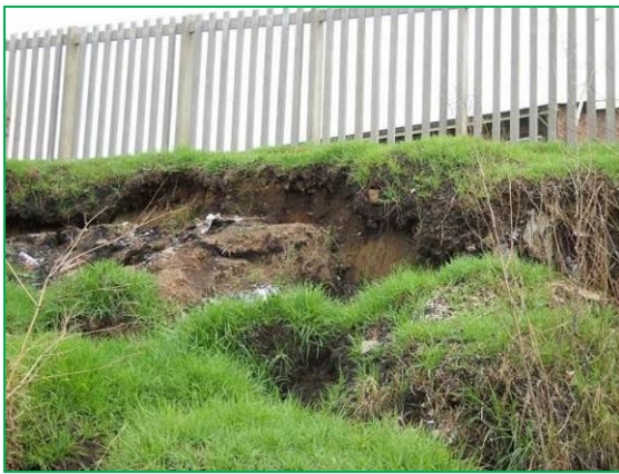
Figure 12: Erosion and bank failure noted within the wetland system.
