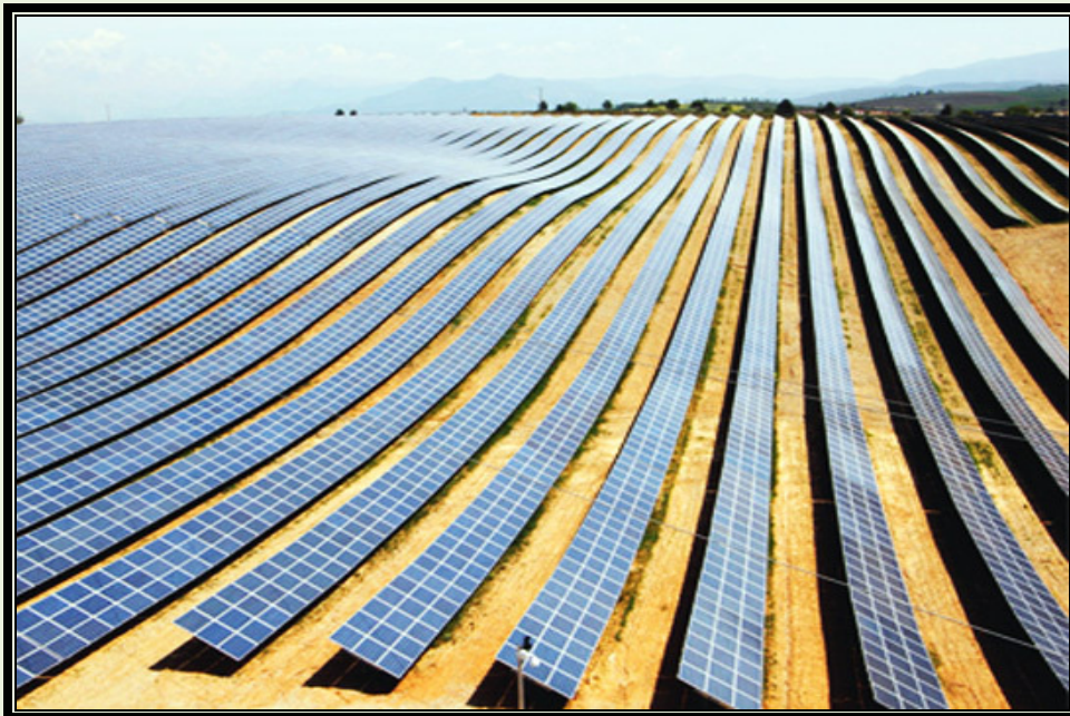
Figure 2: Example of fixed photovoltaic panels.
