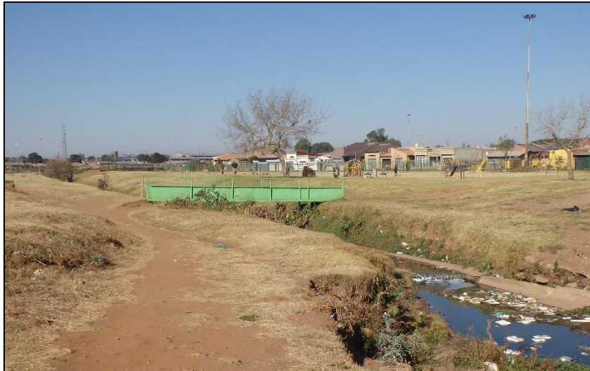
Figure 13: The pedestrian bridge crossing over the river within the study area. Note that the supporting column of this bridge is on the embankment. It is recommended that the supporting columns of the proposed crossings be away from the embankment.
