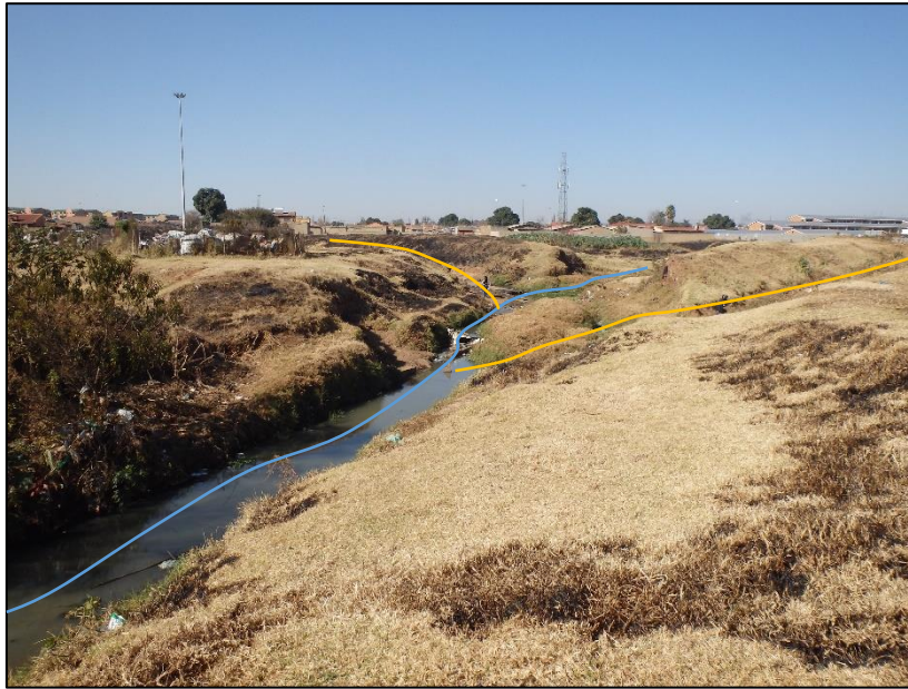
Figure 8: Several stormwater channels (yellow lines) drain into the river system (blue line) within the southern portion of the study area. This has created extensive erosion at the portion where these channels confluence with the river channel.
