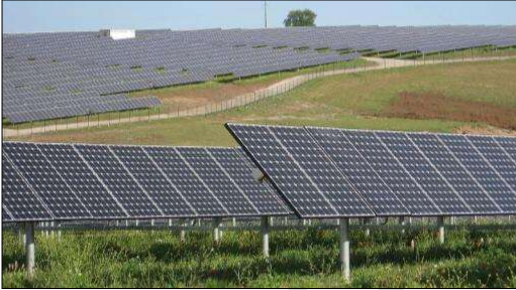
Figure 1-8: View of a Solar PV array
