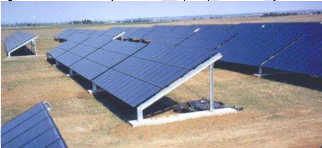
Figure 1-5: Photograph showing the makeup of a photovoltaic array.
