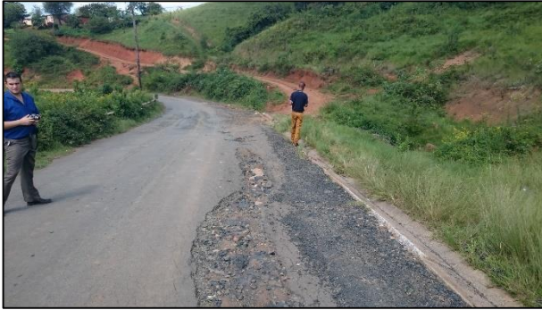
PLATE 13: Deteriorating road surface.
