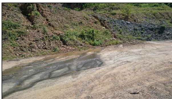
PLATE 6: Deteriorating road surface in the vicinity of the borrow pit. Runoff is flowing over the road surface.
