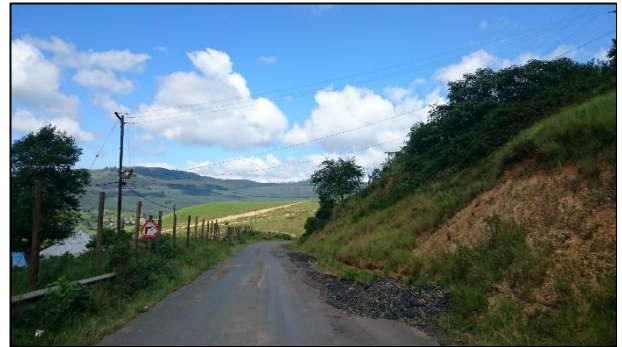
PLATE 10: Deteriorating road surface.
