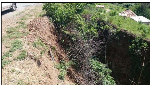
PLATE 5: Deeply incised donga threatens the integrity of the road layer works. The embankment at this site will be stabilised with a gabion retaining structure.
