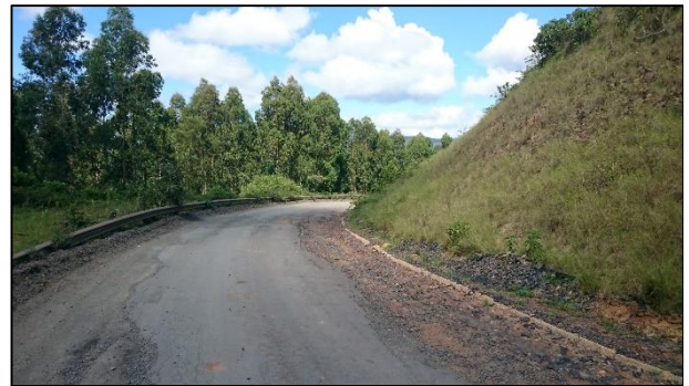
PLATE 112: Deteriorating road surface.
