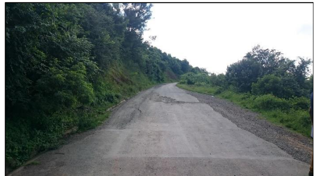
PLATE 148: Deteriorating road surface. Stormwater drainage is to be formalised.
