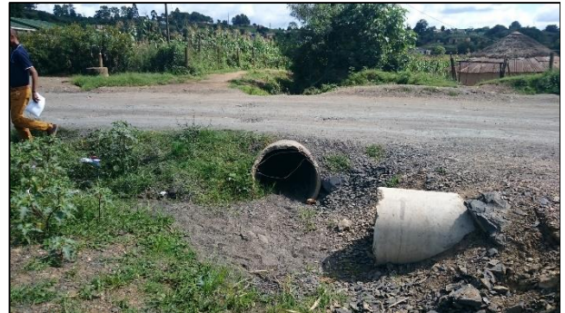
PLATE 22: Culvert will be removed and replaced.
