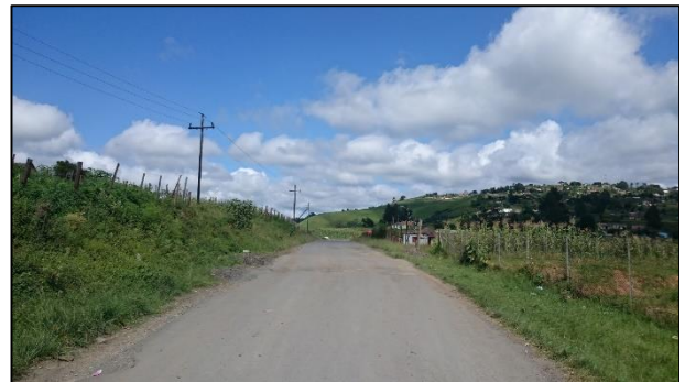
PLATE 24: Deteriorating road. Surrounding landuse is informal housing and subsistence agriculture.
