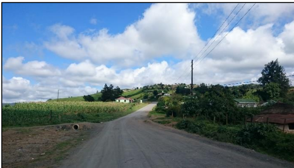
PLATE 23: Deteriorating road. Surrounding landuse is informal housing and subsistence agriculture.
