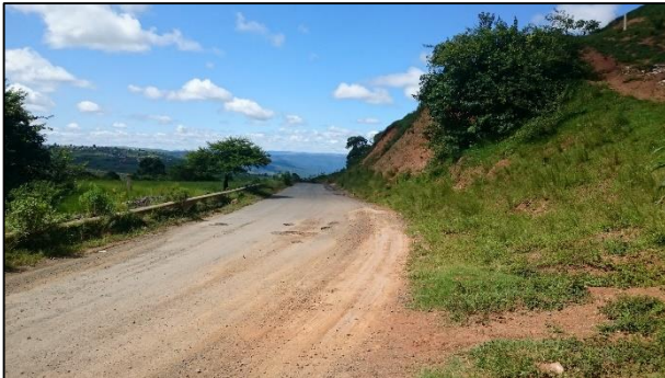
PLATE 15: Deteriorating road surface.
