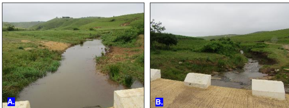
(a): Image upstream of RC68 (b): Image downstream of RC68, showing the structure the pipeline will be tied onto.
