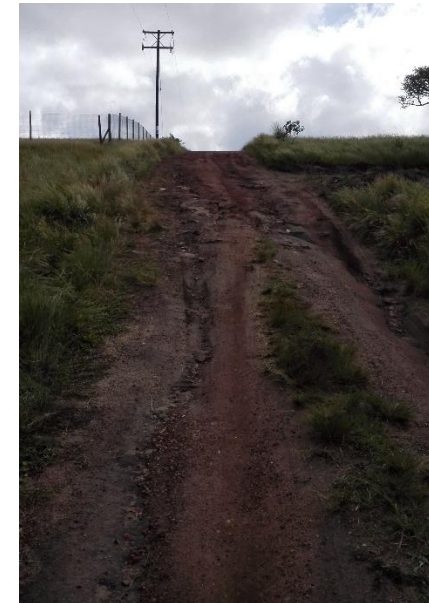
Photograph 8: Shows the erosion at the end of Nositha Road.
