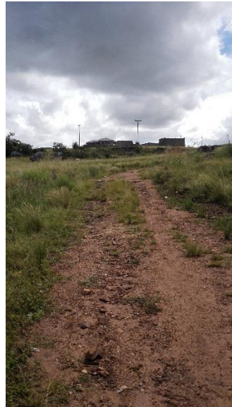
Photograph 7: Shows the erosion at the end of Nositha Road.
