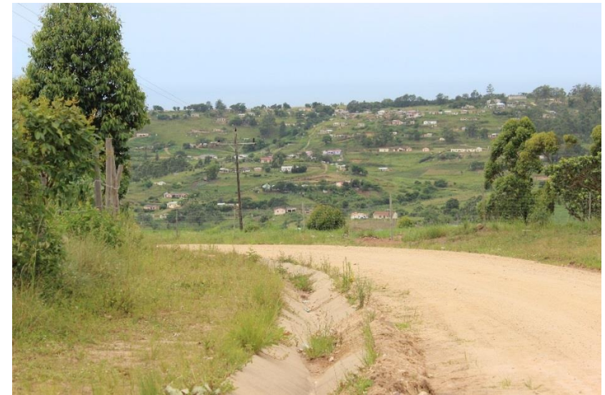
Photograph 4: Shows the existing condition of Nositha Road with storm water drains for 561m along the inner edge.
