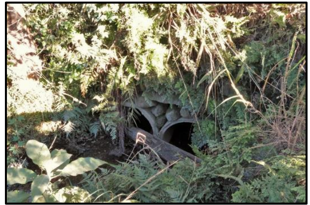
Plate 19. Road D494 stream crossing. Upstream end of the concrete pipes. The bank above them is stabilised by gabions.
