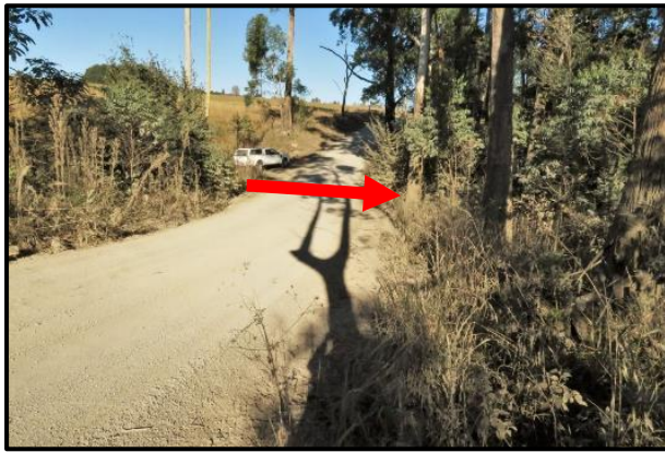
Plate 18. Road D494 stream crossing. Viewed from east to west. The arrow indicates the position of the pipes and the direction of water flow.
