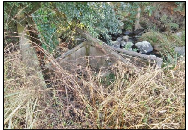
Plate 201. Road D494 stream crossing. Remains of a ram pump support upstream of the crossing
