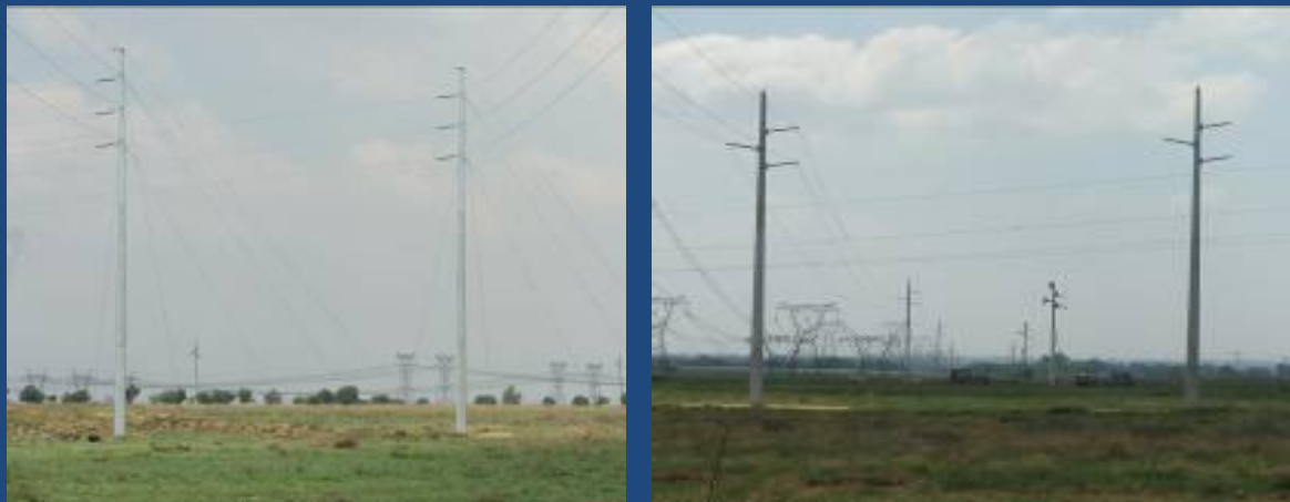
Figure 1: Illustration of the 132kV Pylon Structures (source Eskom)
