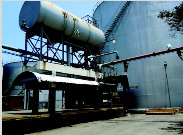
Figure 4: Existing Road Loading Gantry.
