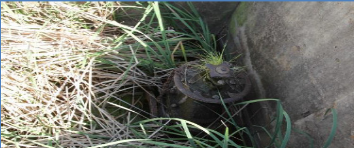
Figure 13: Rietspruit Dam Drain Valve.
