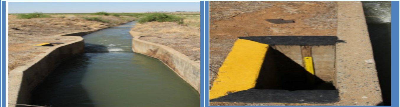
Figure 15: Rietspruit Flow Measuring Gauge.
