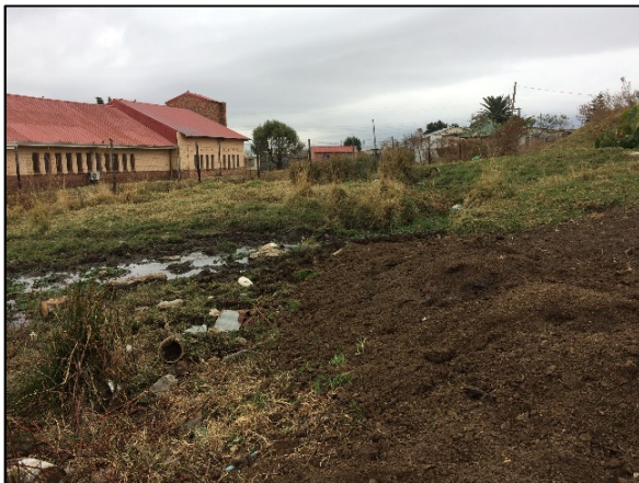
Plate 7-9: Leaking infrastructure evident throughout Wembezi
