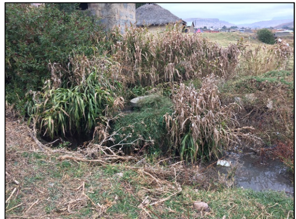
Plate 7-10: Overflowing sewerage manhole, Wembezi as a result of excessive potable water loss
