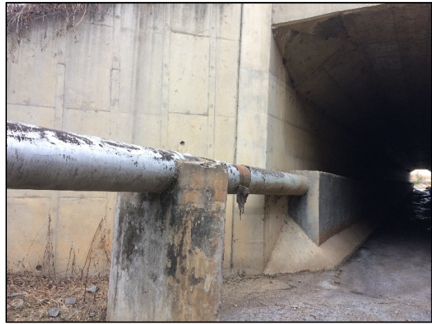
PLATE 4-2: Existing Ø355mm steel rising main aligned through the existing culvert which runs beneath the N3.
