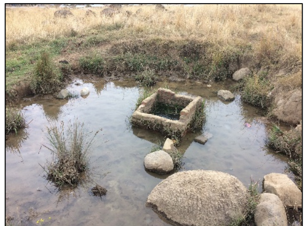
Plate 7-8: Leaking infrastructure evident throughout Wembezi
