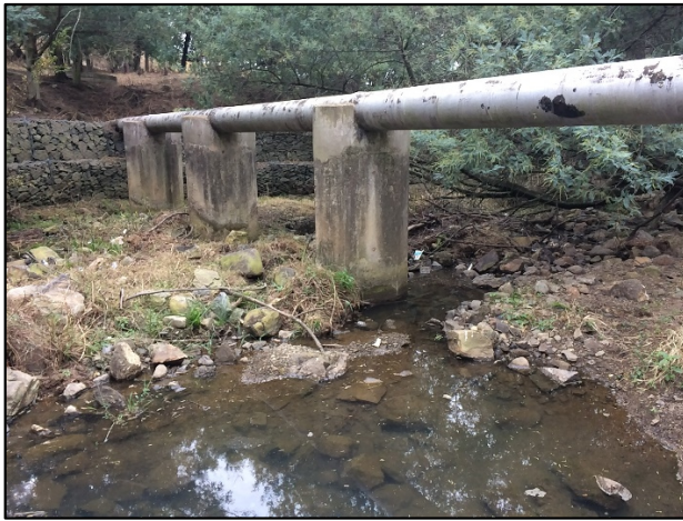
PLATE 4-1: Existing Ø355mm steel rising main pipeline across drainage line below the N3, on existing plinths.
