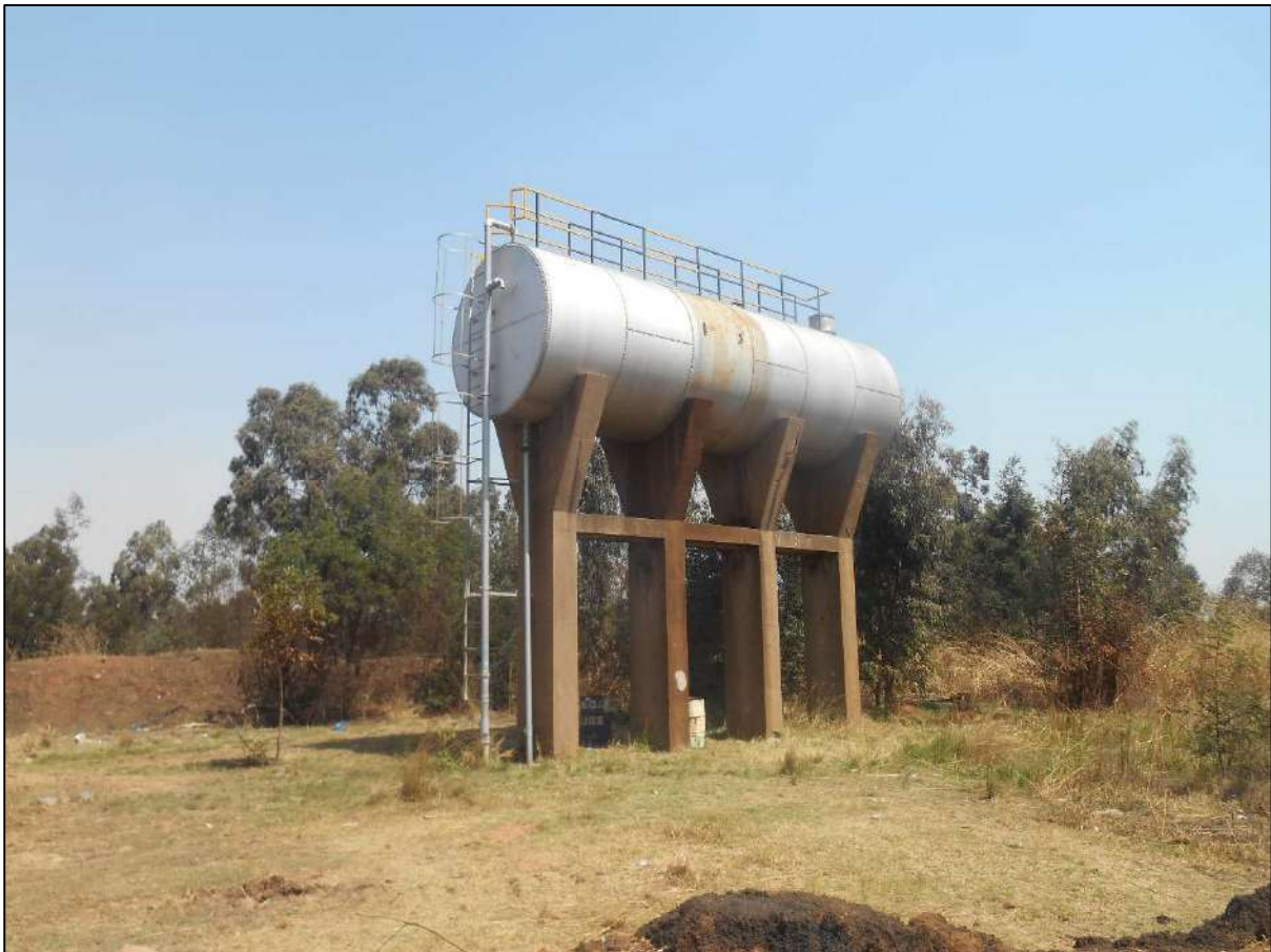
Figure 2: Community Water Storage Tank in Uitkyk
