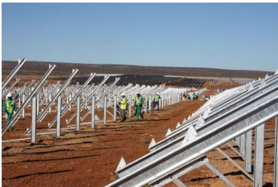
Figure 2.9: Frame, structural details (Lased Solar PV Project, Kimberly, South Africa. Source: Power Technology.com)
