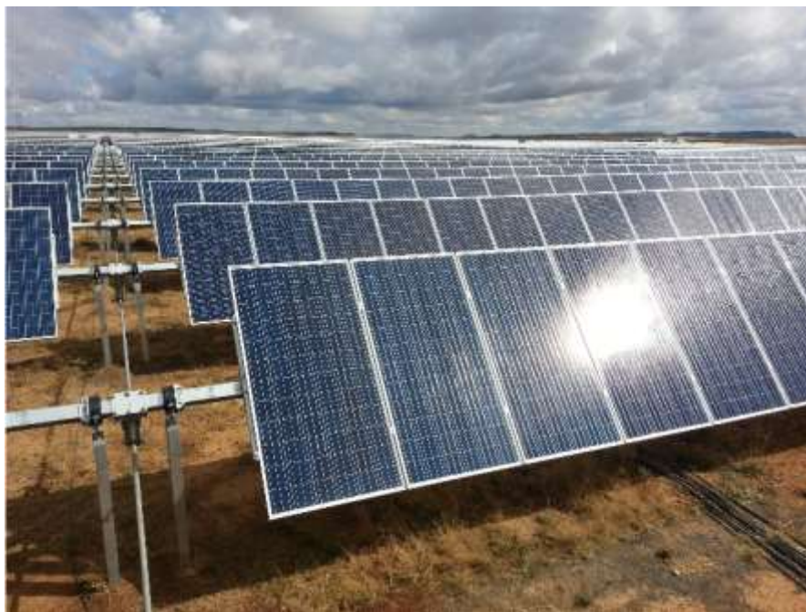
Figure 2.8: The support structures elevate the PV panels and allow for single axis tracking of the sun for increased efficiency (Source: SAPVIA)
