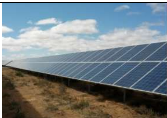
Figure 2.3: Picture of a PV Modules (75 MW plant in Kalkbutt South-Africa Source: SMA)
