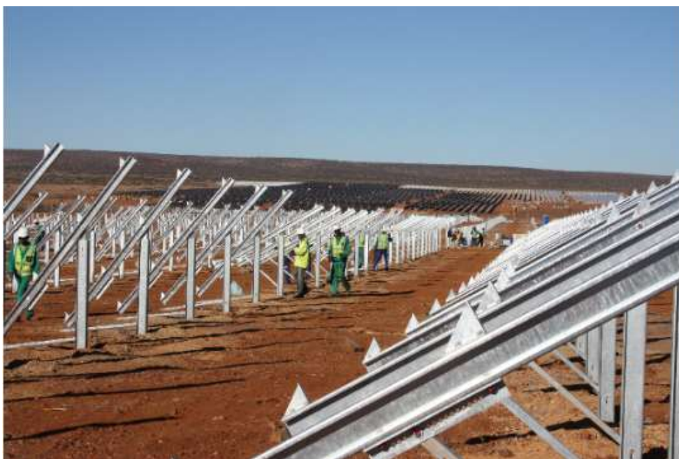
Figure 2.8: Frame, structural details (Lesedi Solar PV Project, Kimberly, South Africa. Source: Power Technology.com)
