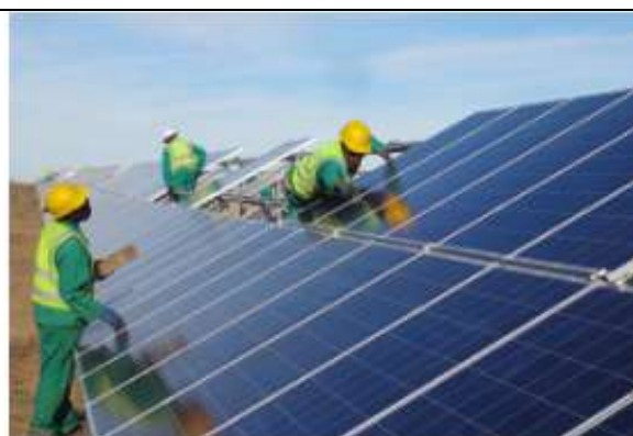
Figure 2.4: Picture of the installation of a typical PV array (75 MW plant in Kalkbutt South-Africa Source: PennEnergy)
