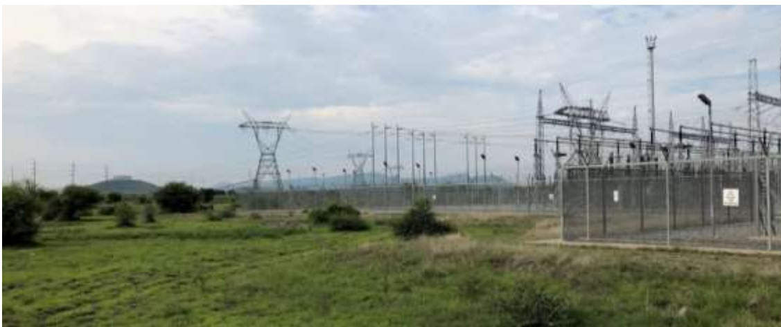
Figure 47: View of Ngwedi Substation at the western end of the power-line corridor linking the SEZ zone and the Ngwedi Substation.
